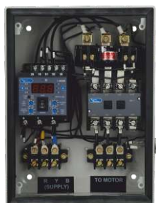
Interior View of MD Starter+ DOL Starter
