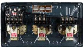
Interior View of MK1 SASD
